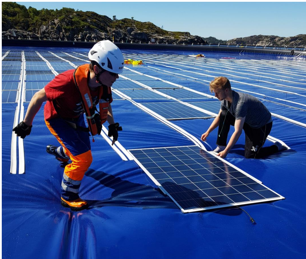
Figure 2.8 Installation of PV modules on the hydro-elastic membrane of the Ocean Sun system (Source: Client, 2021).
