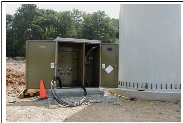
Exhibit 1.5-7 Typical Pad Mount Transformer (shown during construction before terminations landed)
