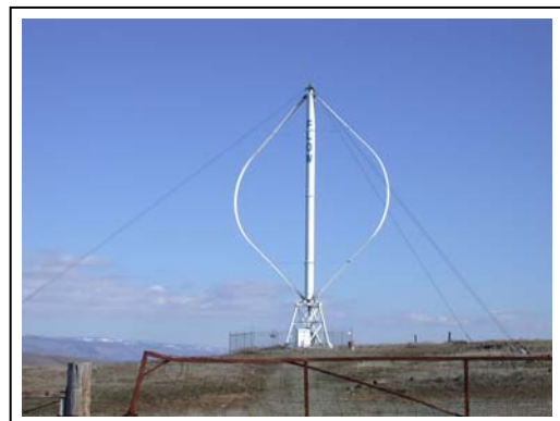
Exhibit 4.5-2 FloWind Vertical Axis (Darrieus Wind Turbine) Located on Thorp Prairie, near Ellensburg, WA
