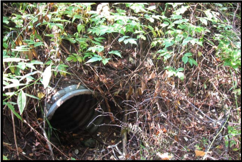
CV1173A-ST facing South
