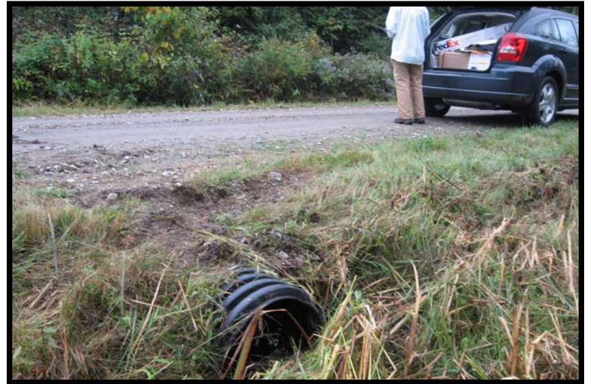
CV1172A-ST facing South
