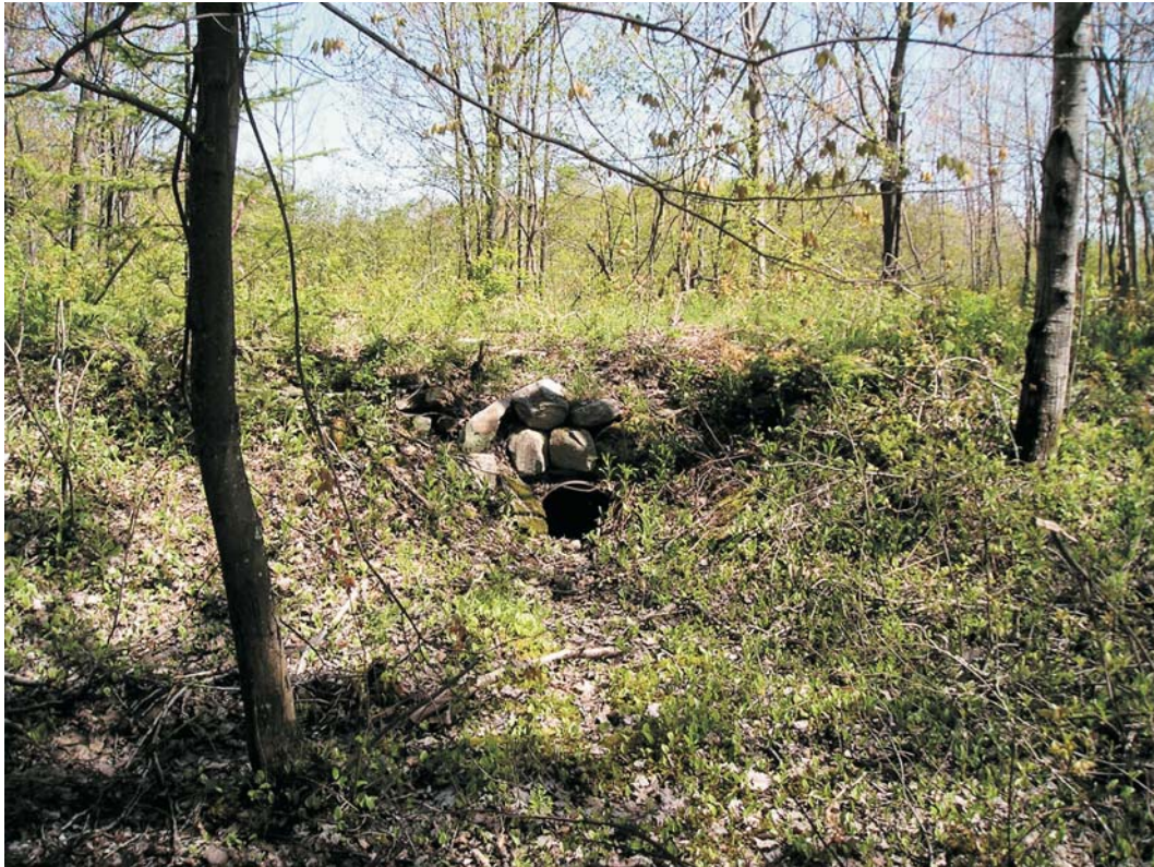
Photograph 19. Culvert showing the profile of the berm for the abandoned paved road in the southern part of the Clinton Mills Site; view to the north.
