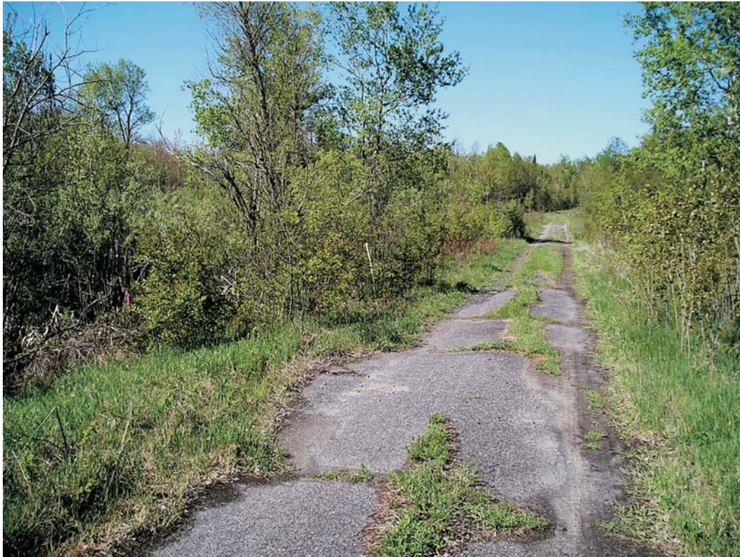
Photograph 17. Existing conditions of abandoned paved road within the southern part of the Clinton Mills Site; view southwest.
