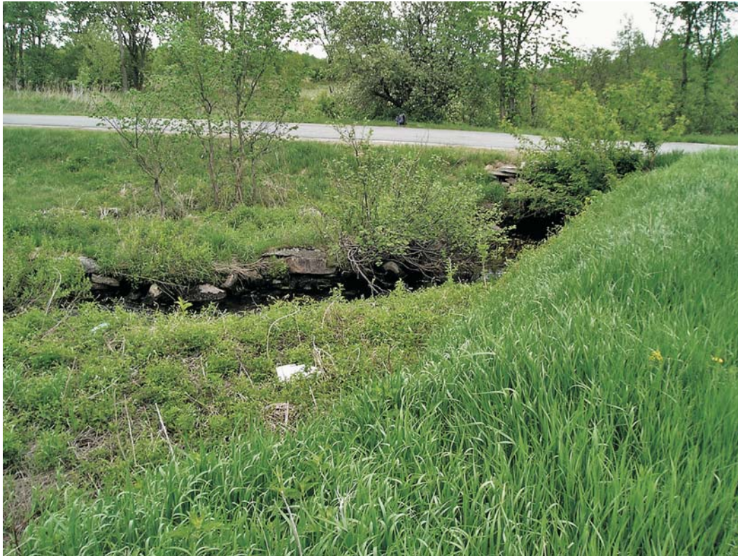
Photograph 15. Channeled and culverted stream under Rogers Road – note profile of O&LCRR berm at right; view to the east.
