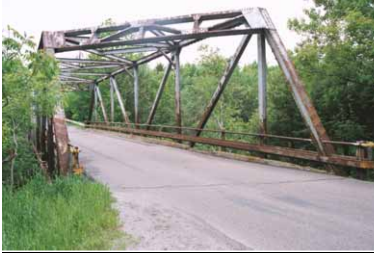
Vertical clearance limitation
