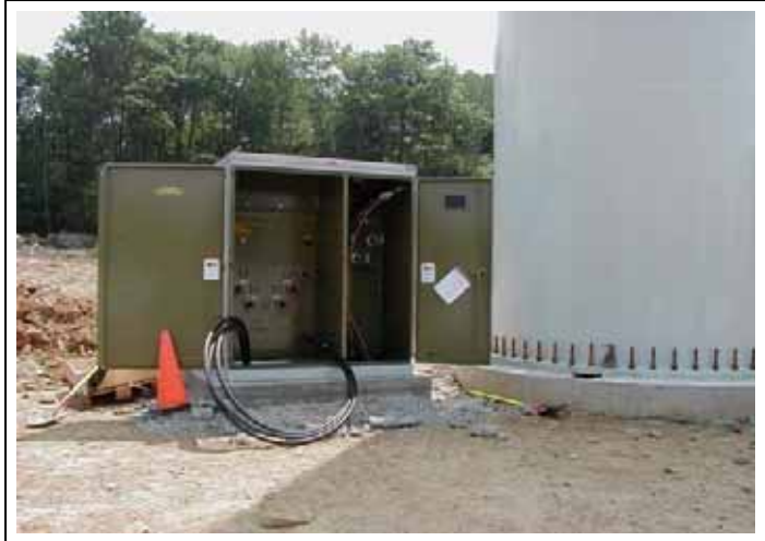
Exhibit 1.5-7 Typical Pad Mount Transformer (shown during construction before terminations landed)
